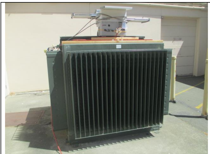
17. View of the pad-mounted transformer.
