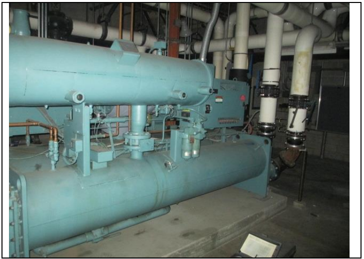
8. View of a chiller unit.
