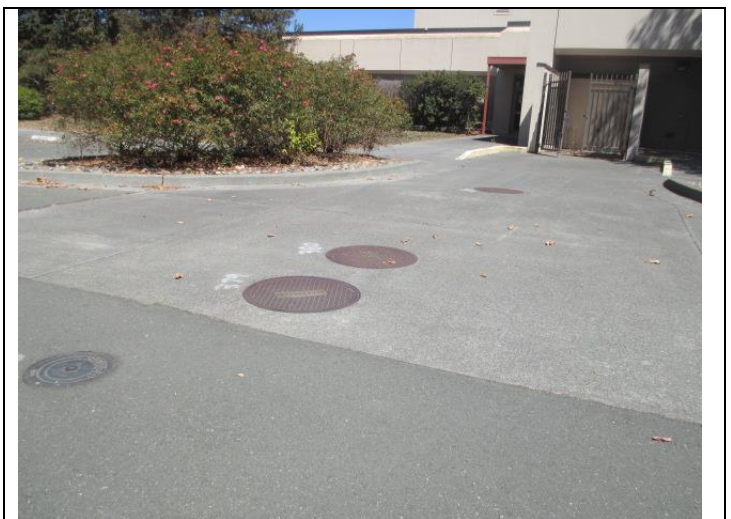
18. View of the grease interceptor system.
