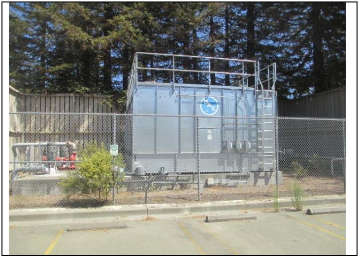
16. View of the exterior cooling tower.
