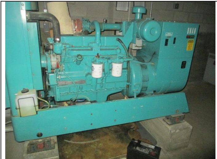
9. View of the emergency generator.
